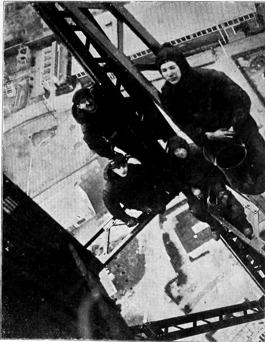
A SURE FOOT AND STEADY NERVES ARE REQUIRED BY THESE WORKMEN REPAIRING AND PAINTING THE GIANT ANTENNA TOWER OF A BERLIN STATION. MOST PERSONS GET DIZZY JUST LOOKING AT THE PICTURE.
