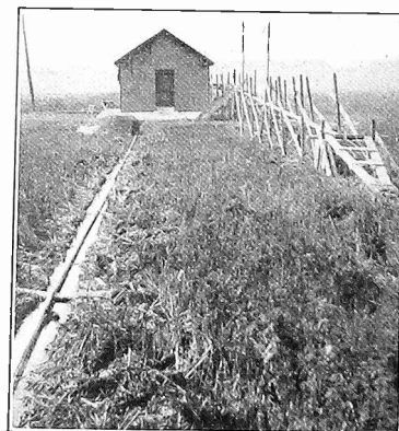
AN UNDERGROUND antenna will be used by WGL at its new location in Seacaus, N. J. Here it is shown just prior to submergence.
