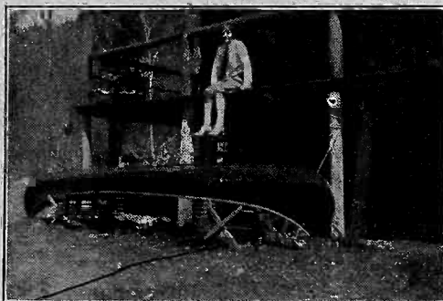
THE FIRST step in installing an underground antenna. It is laid upon the ground. The earth is then dug up and the wire buried.
