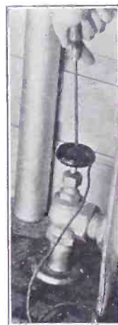
The trick shown in the photo utilizes the natural obstinacy of water in refusing to travel uphill. "High and dry" is a good slogan for the connection.
