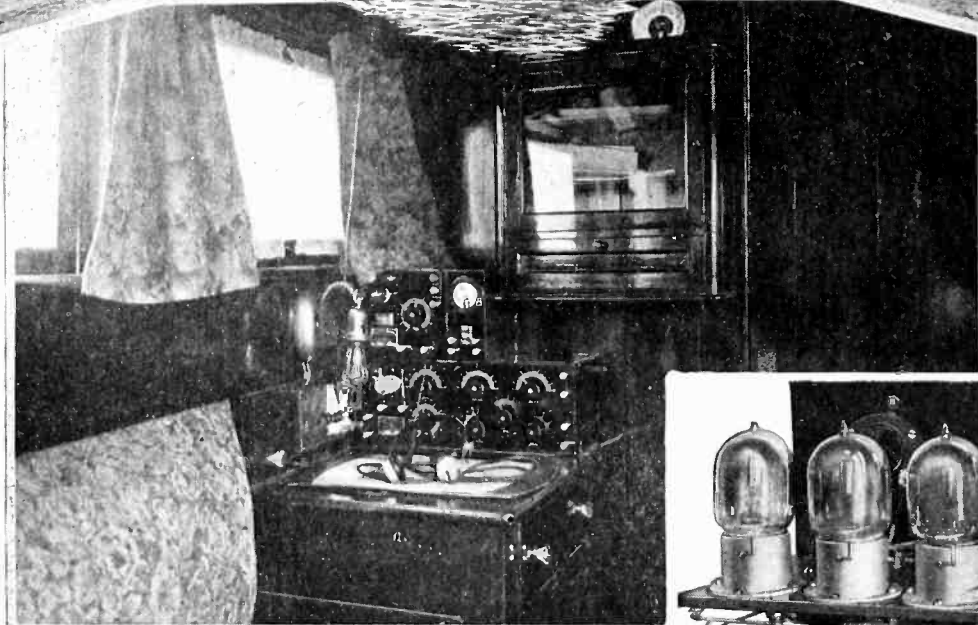
The accompanying views of the Vacuum III show a model boat installation. It takes up very little space
