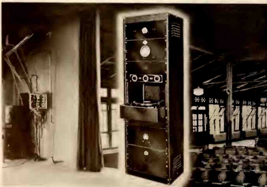
The medium sized auditorium on Welfare Island, N. Y., has amplifier, tuner, and phonograph equipment installed on the stage.
