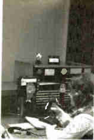
A microphone at the switchboard permits our company operator to page people simultaneously in both buildings.
