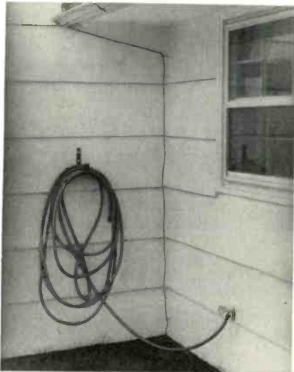
Fig. 6—Shielded coaxial cable can be run directly adjacent to aluminum gutter without fear of mismatch.
