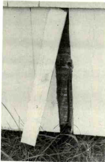
Fig. 7—Coax download is fed into house under shingle, making neat, unobtrusive installation.
