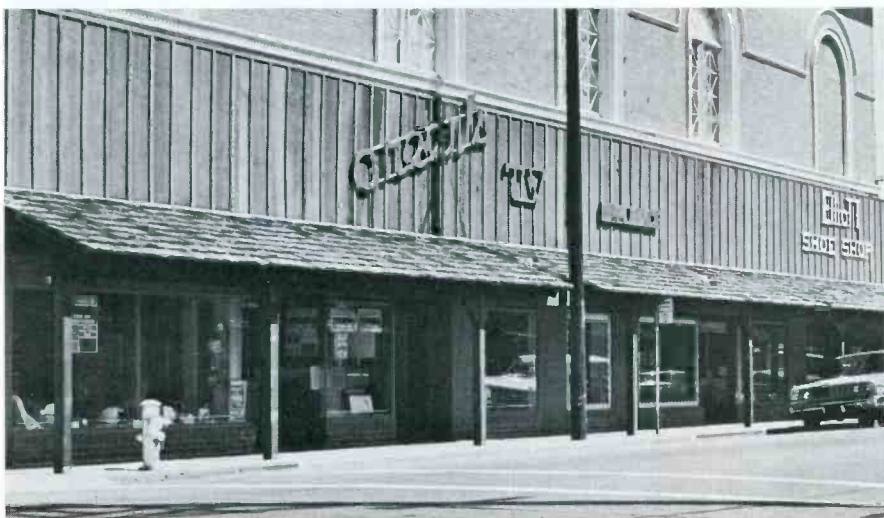
Remodeling of store fronts in Antioch is reviving business. Mr. Green spear-headed the modernization program.
