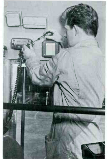
Two-way communications technician installs control unit in a public bus. Courtesy G-E.
