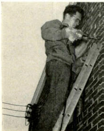
Fig. 2—Ladders should not be placed where they can fall across power lines.
