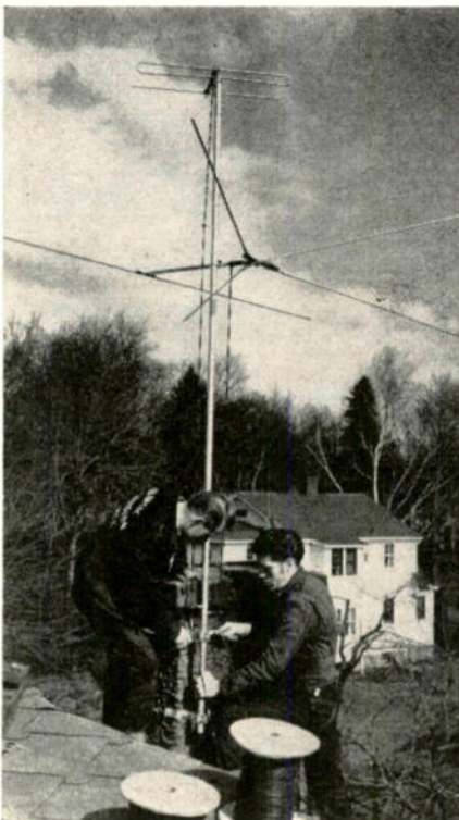
Fig. 4—Team work shortens installation time. A spintite or open-end wrench is advisable, replacing pliers used in this illustration.
