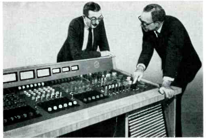
A 6ft console controls audio for the 800-seat Circus Maximus supper club in Las Vegas.
