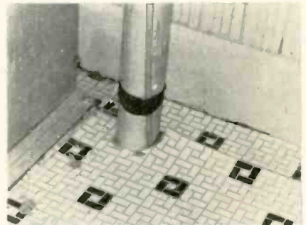
Fig. 5—Taping line to pipe results in signal attenuation (shunt capacity) and mismatching.
