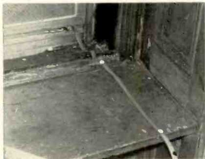
Fig. 6—Storm or other metal windows can mismatch line, as well as tacks shown on line.
