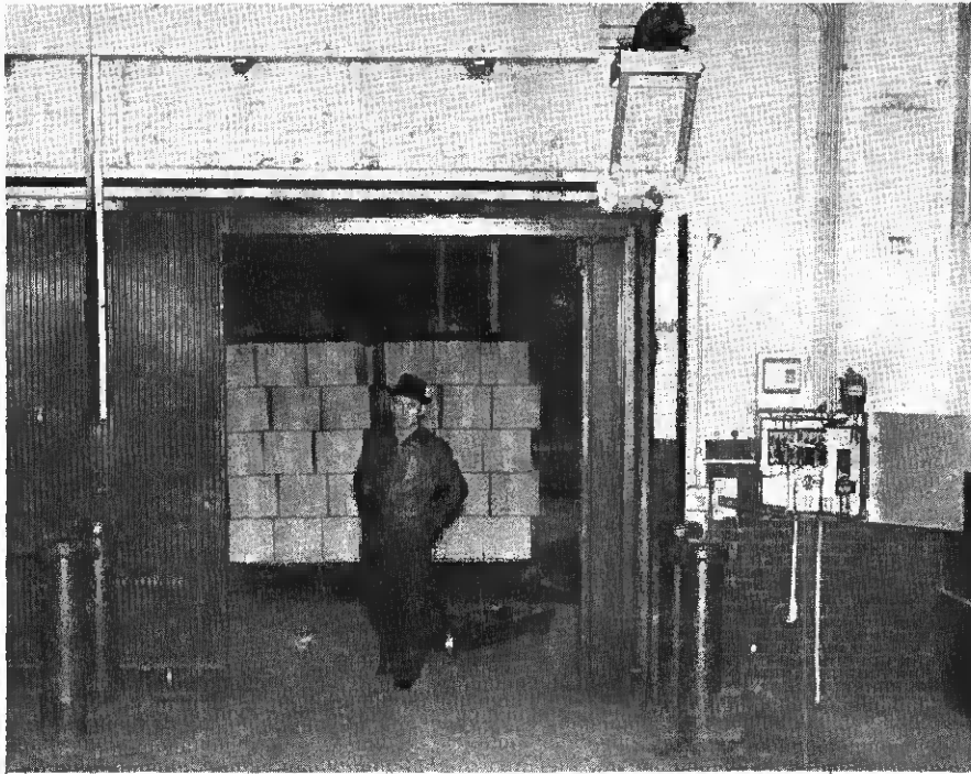
GE photo-cell door saves time and heat at a big Louisville, Ky., tobacco plant. A hinged section and limit switch reverse motor if any person is caught in door.
