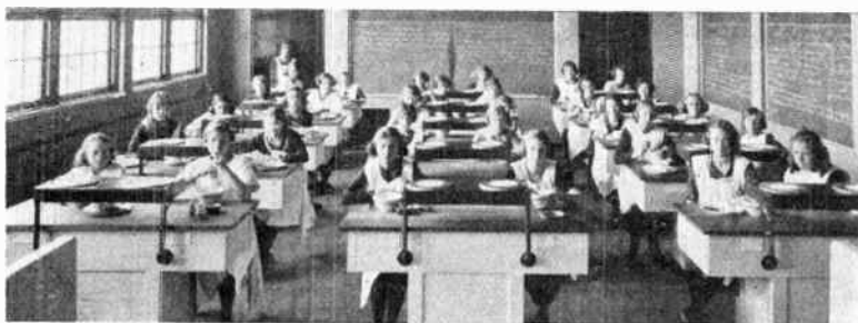
Thirty-two hot plates and one electric range comprise the electrical installation in the domestic science department of this Ogden, Utah, high school.
