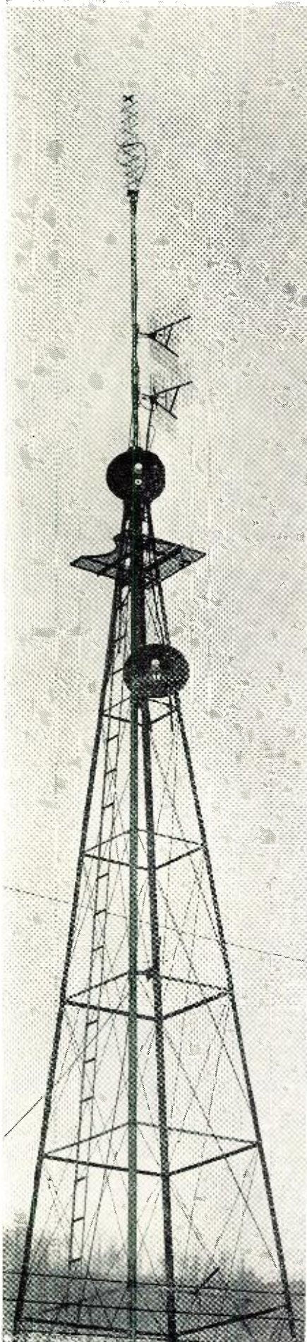
← Fig. 6. Tower and transmitting antenna for channel 82 satellite located in town of Emporium, Pa. The channel 22 booster corner reflector antennas and parabolic antennas for microwave links are also shown.
