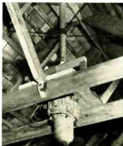
Fig. 2. A pipe shaft runs up through the roof inside a larger pipe bushing, steadied by pipe straps. At the top are two 2 x 6 roof supports. Note the BX cables.
