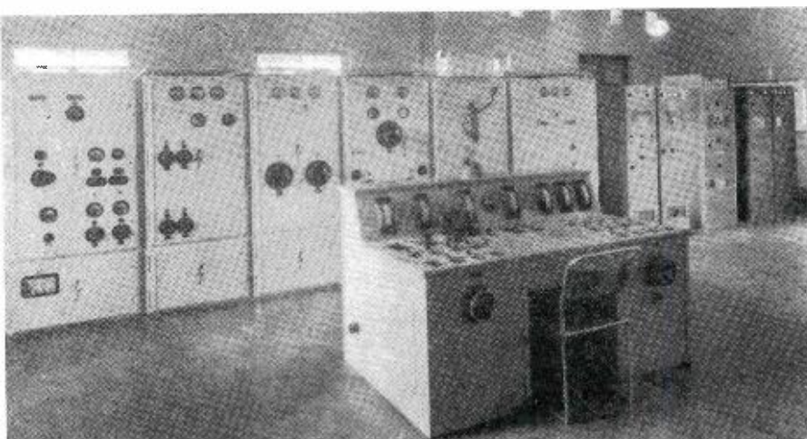
Transmitting equipment of the Radio Clube de Mozambique, Lourenco Marques, Mozambique. Two additional transmitters, a 7 kw. and a 5 kw., are now on order from RCA.
