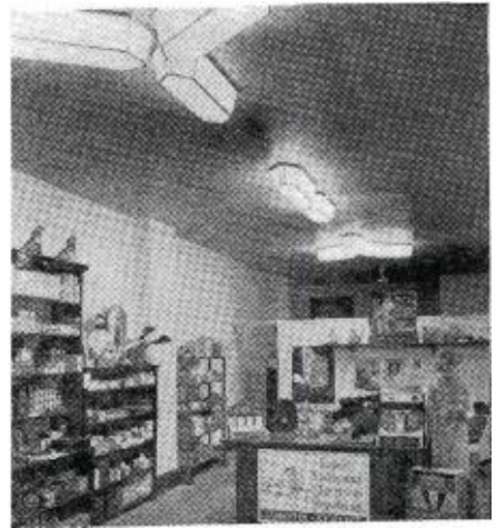
Because of their flexibility, the new fluorescent lamps are adapted to many different types of installation. In this radio and electrical repair shop, luminaires of modern design serve both decorative and functional purposes.
