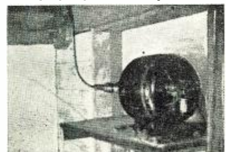
Motor turns array by means of flexible coupling to gear box. \frac{1}{2} hp. is used.
