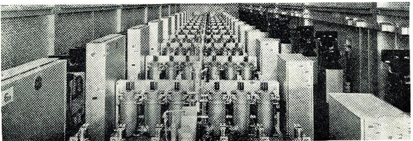
Twelve-unit ignitron mercury-arc rectifier installation in a large electrochemical plant.
