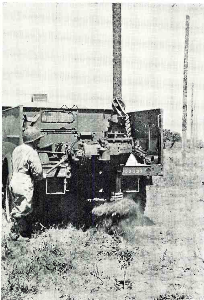
A powerful post-hole digging machine, capable of digging thirty holes an hour, can be operated by a two-man team.
