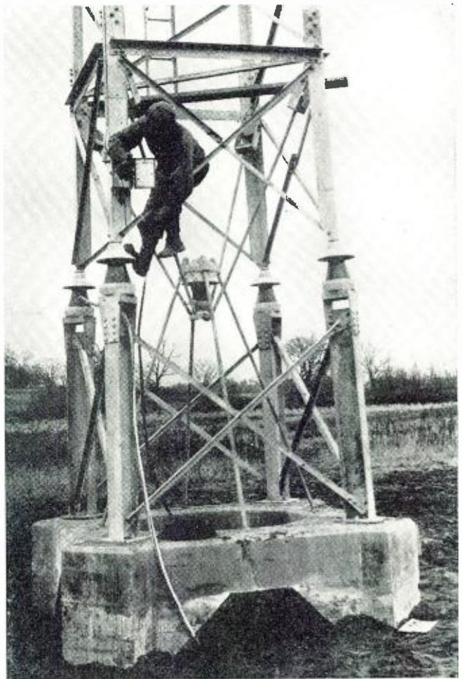
Installing power wire on a Department of Commerce airways radio station antenna tower. Note the concrete base.
