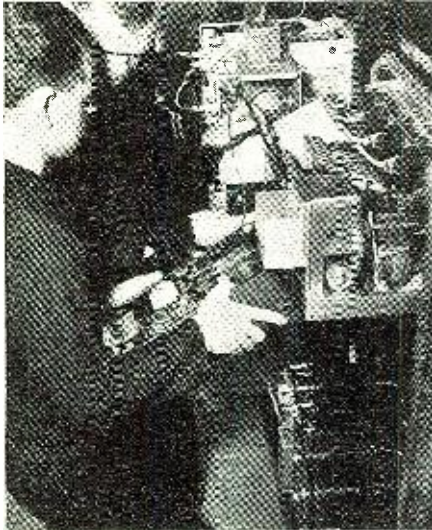
Checking contactors on beacon unit.
