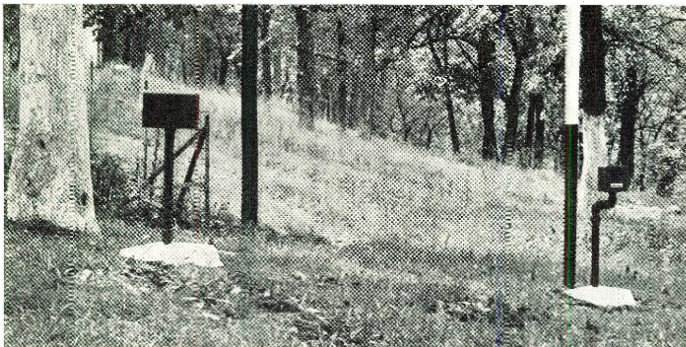
Here is a typical outdoor installation of photocell light source and receiver.
