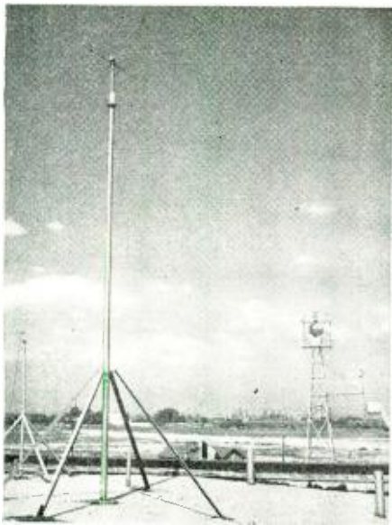
Fig. 8. UHF Airport Traffic Control Antenna System at large Eastern Airport.
