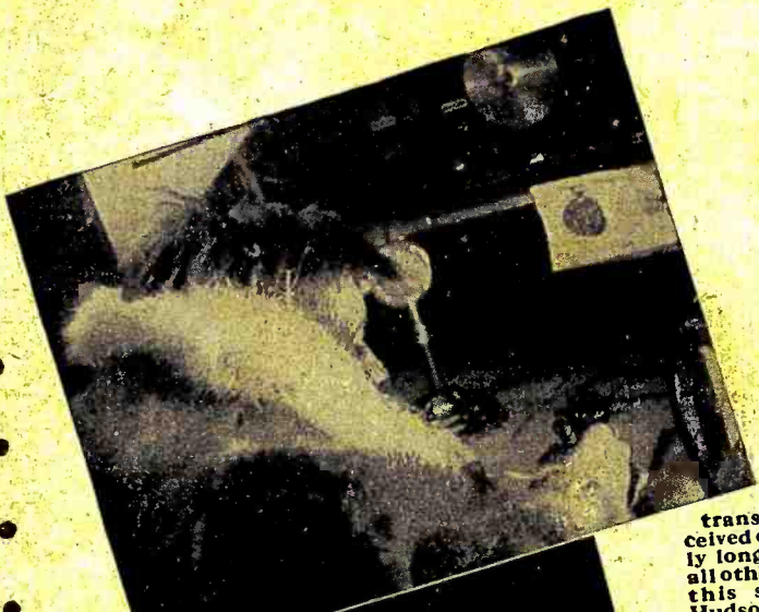
THE CONTROL BOARD OF WFBR, NBC station, of Baltimore, Md., showing panel installation of 1938 Super Sky rider.
