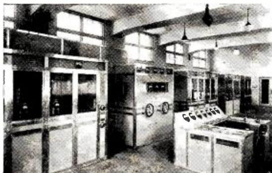
VIEW OF TRANSMITTER ROOM
