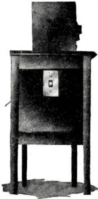
Fig. C: How the two-way switch shown in Fig. 3 is mounted on the side of the cabinet holding the radio receiver.
