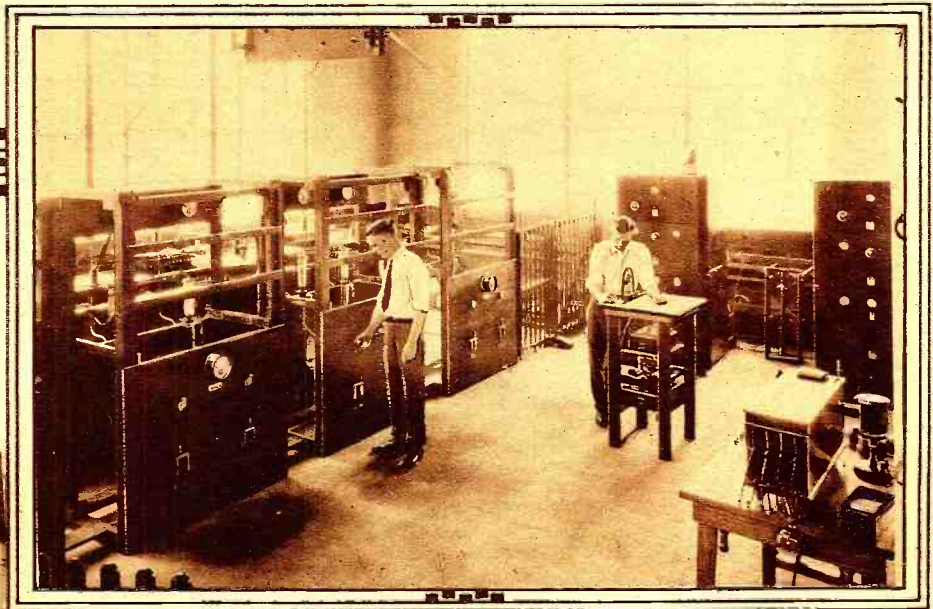
THE SUPERPOWER TUBES. These three units house the water-cooled tubes with their attendant step-up tubes and transformers. The two solid panels at the side are the terminal boards for the land lines that come from the studio in Schenectady.
