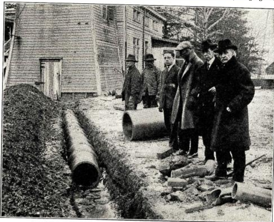
Laying of terra cotta pipe, in which is placed copper tubing, and the whole is covered in four feet of soil. These underground antennae, each 100 feet long, extend north, south, east, and west respectively.
