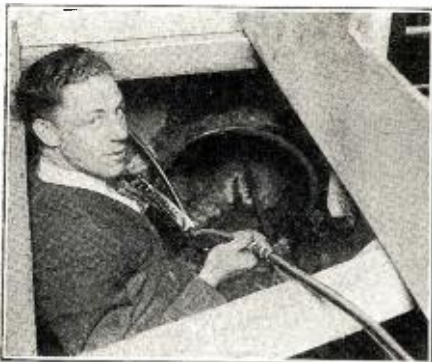
Unusual photograph of making connection of transmitter with underground antenna. The copper tubing is placed in the terra cotta pipe.
