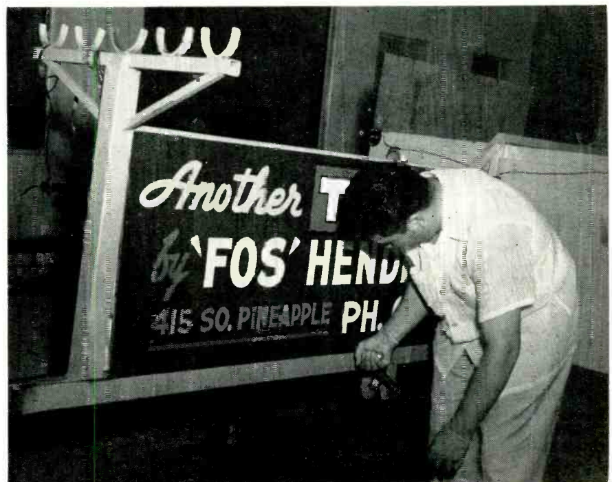
• The first section of the mobile demonstration antenna is cranked up by hand. The total height of the antenna tower is sixty feet. As a sales aid, it answers initial reception question and clinches sales in one Florida fringe area.
