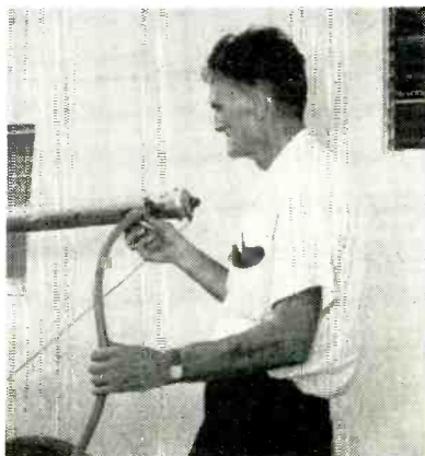
• Water pressure is used to boost the top two antenna tower sections into position.
