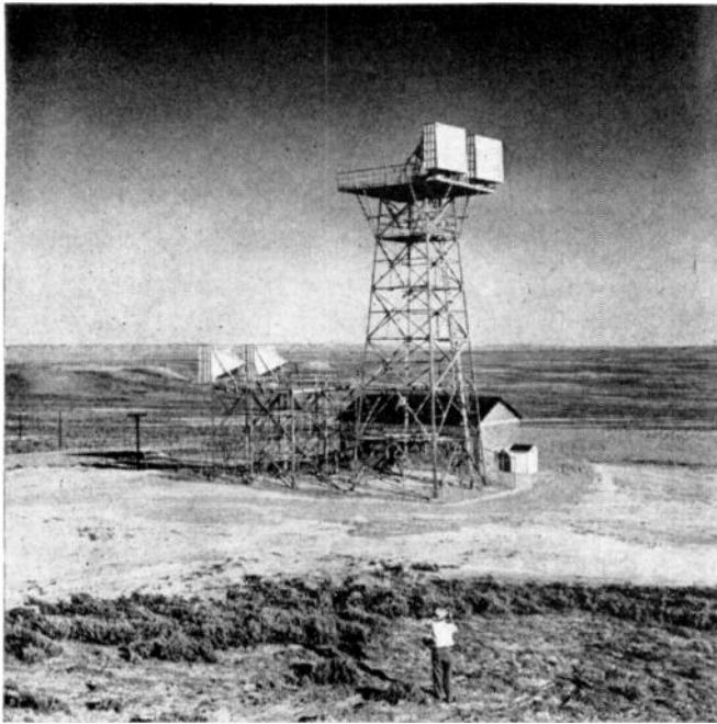
• A link in the A. T. & T. system at Creston, Wyo., showing receiving and sending microwave antennas at two levels.
