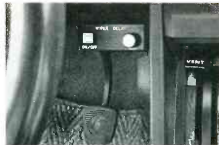
FIG. 5—THE INSTALLED SOLID-STATE WIPER CONTROL under the dash. Here, the holes for the lid were drilled out, and 4-40 screws were used to mount the case under the dash. You can also use the lid, and attach the case with Velcro or double-sided tape.
