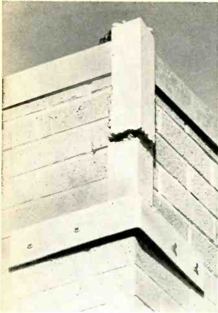
Mounted on the four corners of the building, the posts anchor guys firmly.
