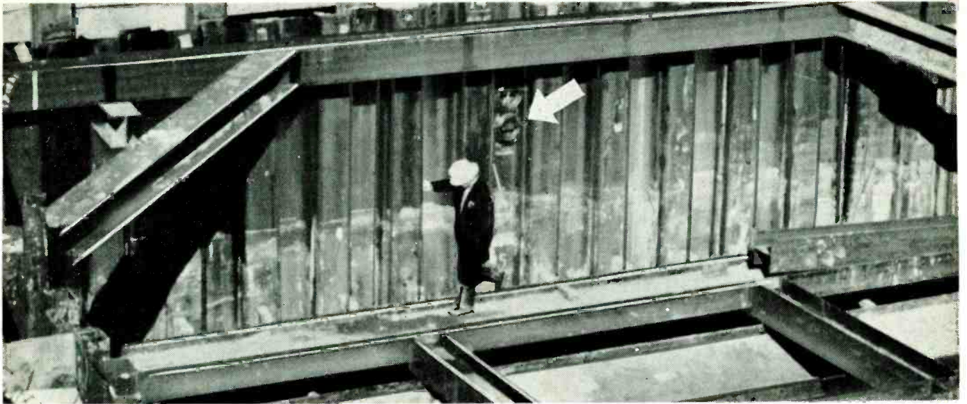
Massive steel cofferdam, braced with I-beams, holds walls of this excavation and keeps them from caving in. Pressure cells fitted to beams can warn of excessive stress before a cave-in occurs.
