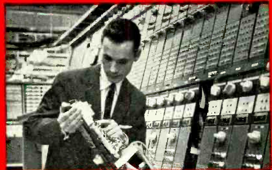
Checking panel wiring of Simplex console
