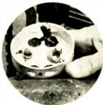
Where cable enters tapoff box the braid and insulation are rolled back to form grommet—joint then made weathertight.
