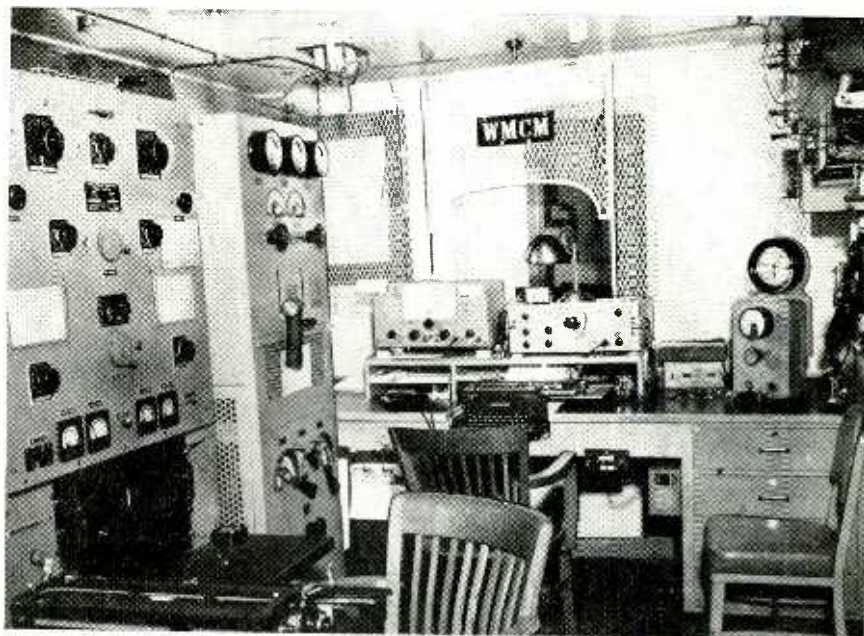
This installation is in the radio room of the Moore-McCormack liner Uruguay .
