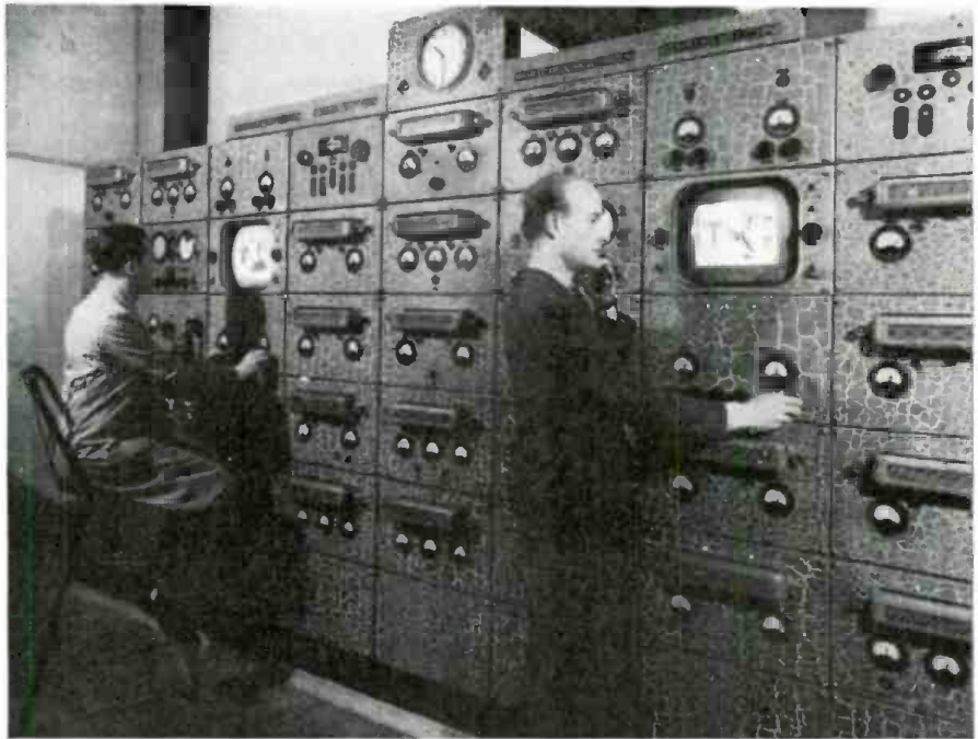
France's only television transmitter is in base of Eiffel Tower. This is the control room.
