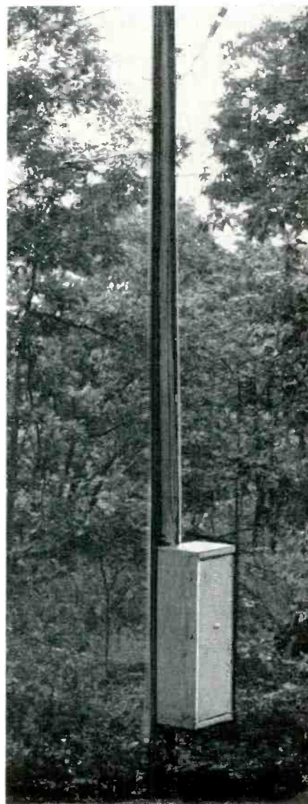
A typical RCA "pole mount" installation.
