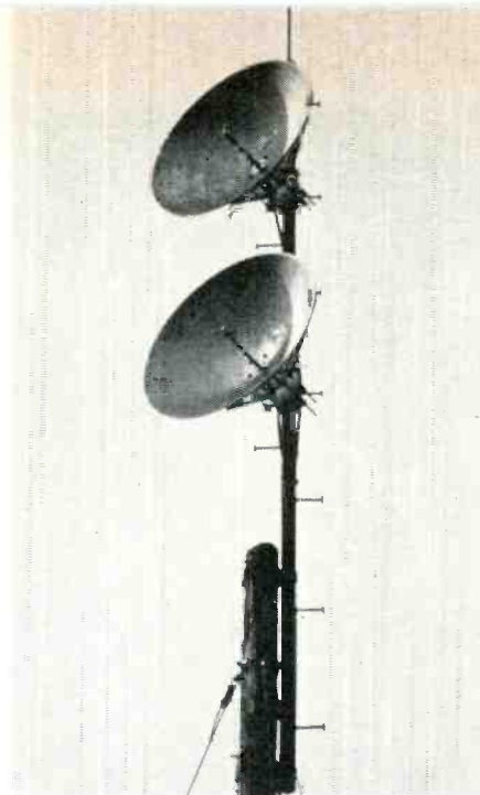
Dipoles with parabolic reflectors provide the best antennas. Opposite polarization is used for transmitting and receiving.
