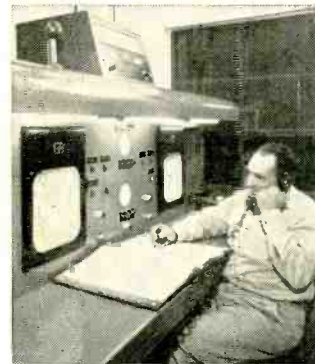
Operator at control console at regular pump station also controls remote stations. Telemeter charts provide continuous record of both local and remote station operation over 24-hour period
