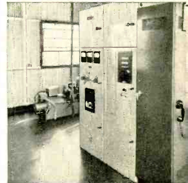
Remote-station control building contains radio cabinet (right); cabinet for relays, switches and starting equipment (center); controls for local operation (left). Stand-by generator is in background
