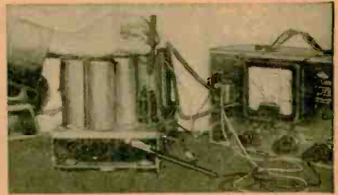
Photo 5—Grid to ground shows a dead short.
