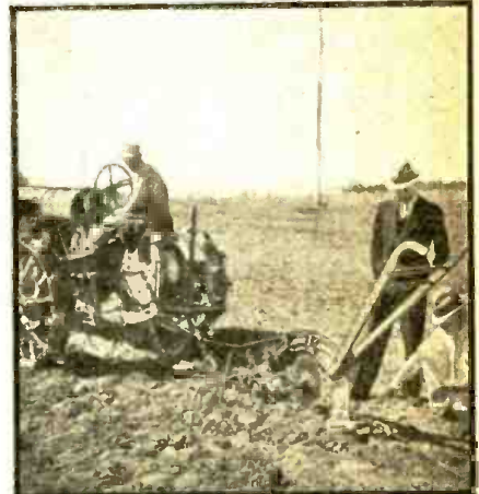
Laying 50 miles of copper wire which is an unseen factor in the efficiency of the new KDKA antenna; it is buried about a foot deep, to form a ground. In the background, masts of KDKA's multiple system.
