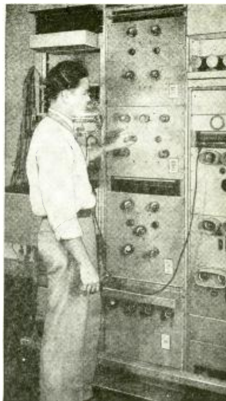
Fig. A The device under trial in the long-wave transatlantic telephone channel is shown here.
