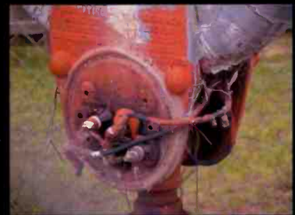
Here is a case of a missing terminal cover leaving tower lighting connections exposed
