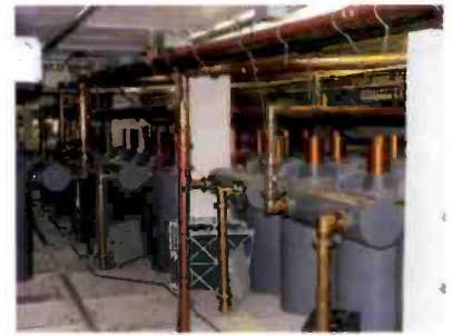
A portion of the 10 station ERI combiner in Seattle
