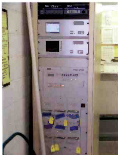
Entercom's KBSG/97.3 HD Rig A BE 201 running ~ 700 watts.
