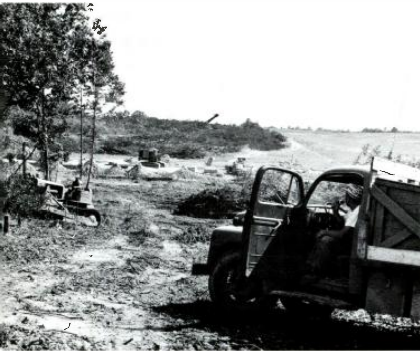
Mobile radio speeds site clearing for new highway as truck driver (foreground) calls his foreman in radio-equipped vehicle several hundred feet away for instructions, and gets them immediately.
