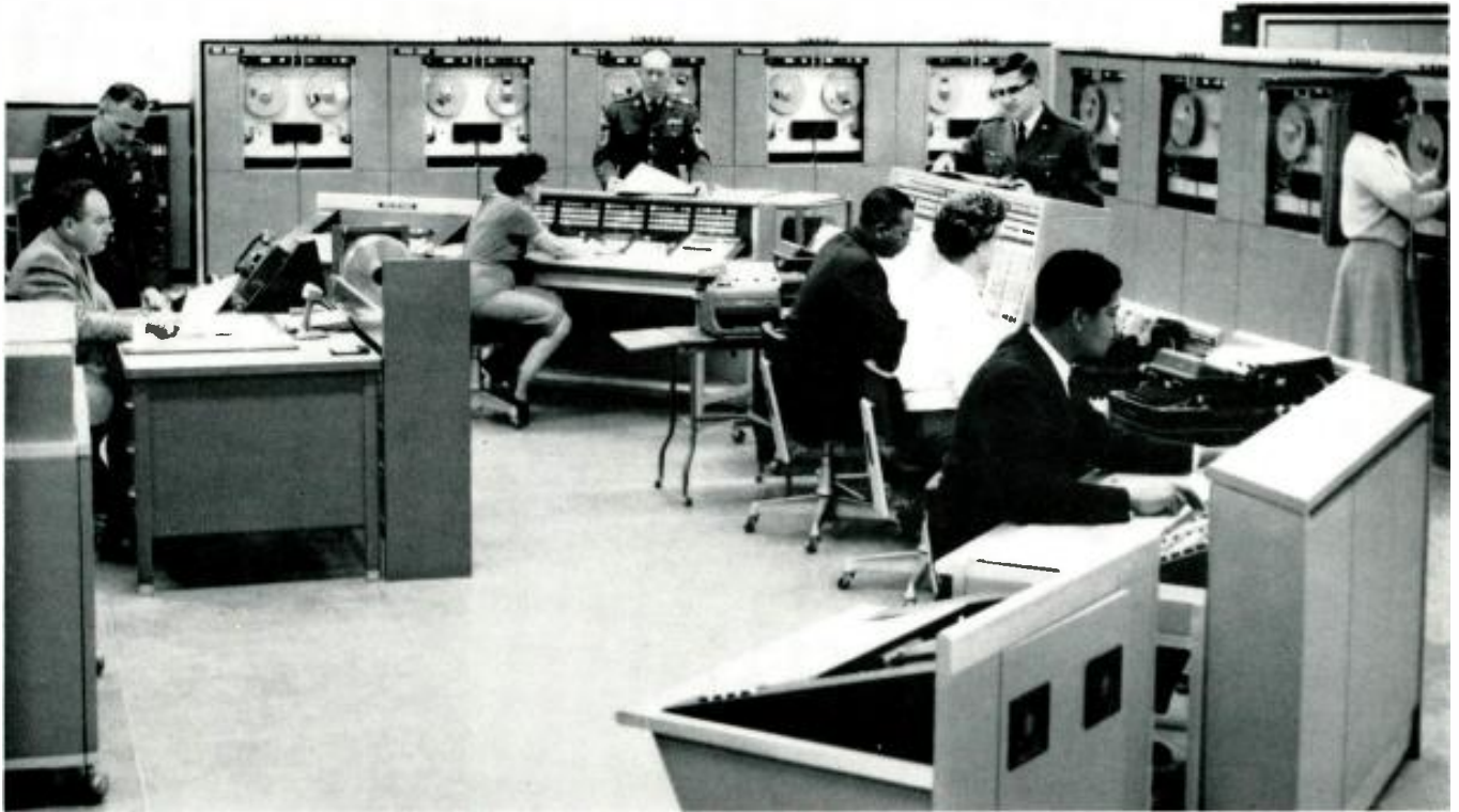
This automatic electronic DATACOM/AUTODIN switching center at Andrews AFB relays data electronically at speeds of from 100 to 3,000 words per minute between more than 300
