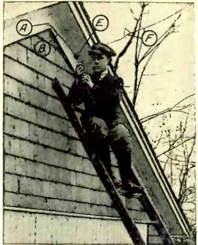
II Fastening the far end of the antenna through the metal eye of the insulator. A is the screw eye, B a piece of rope, the insulator and F the antenna wire.
