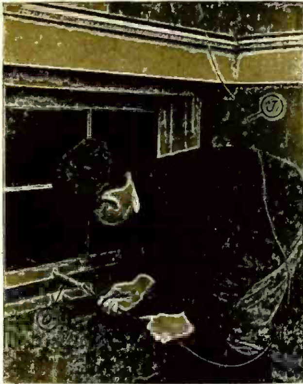
III The insulated lead in wire is brought into the house through a porcelain bushing pushed through a hole drilled in the window sash.
