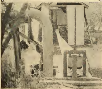
Motor Belted to a Vertical Pump
