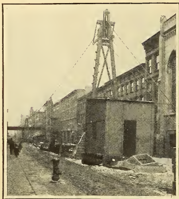
Aerial Cable Way a Block Long. Motors for Hoisting are Housed in the Stackless Shanty
