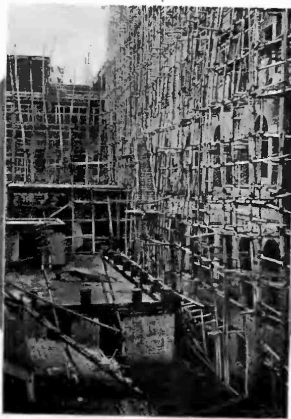
The Ancient and the Modern Methods of Building Construction: In the Upper Left Hand Corner is seen the Structural Iron Work, and at the Right, the Native Bamboo Scaffolding.
