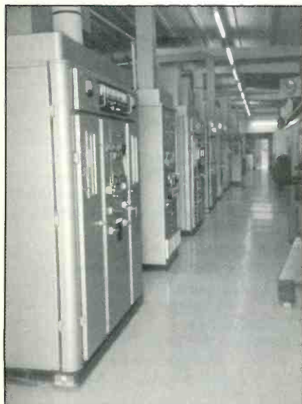
"Transmitter row" at the Caribbean relay station on Antigua which relays BBC and DW programming.
