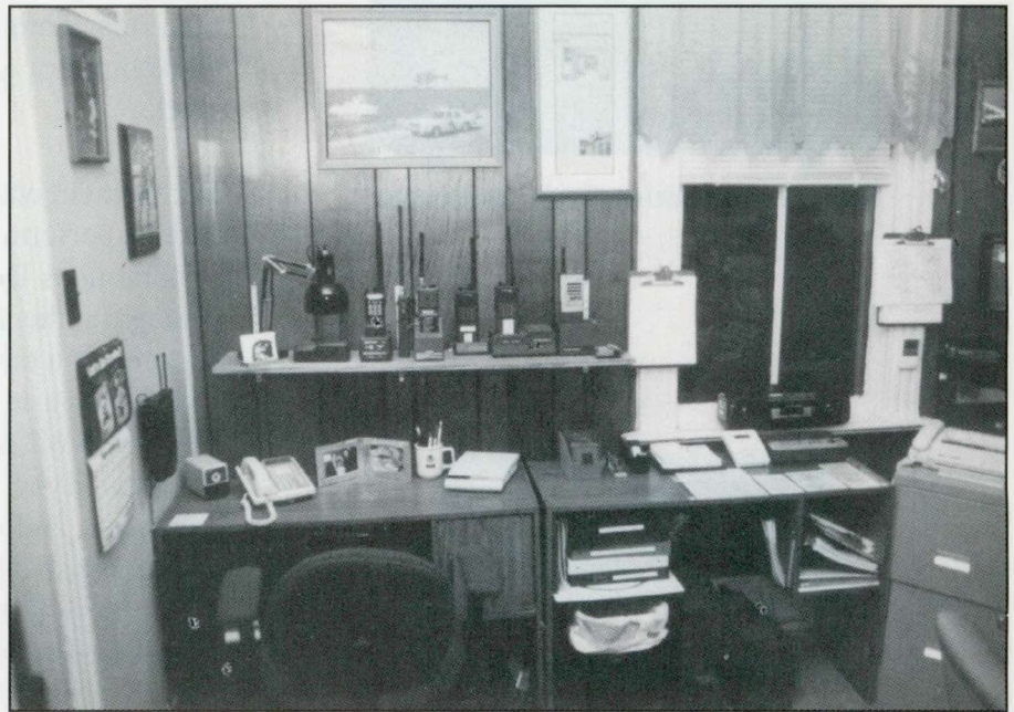
Harrison Weather Center (HWC) first floor equipment includes backup communications equipment and WTs. There are WTs for low band, high band, UHF/GMRS, T band, and amateur radio repeater access for SkyWarn coverage and disasters.
